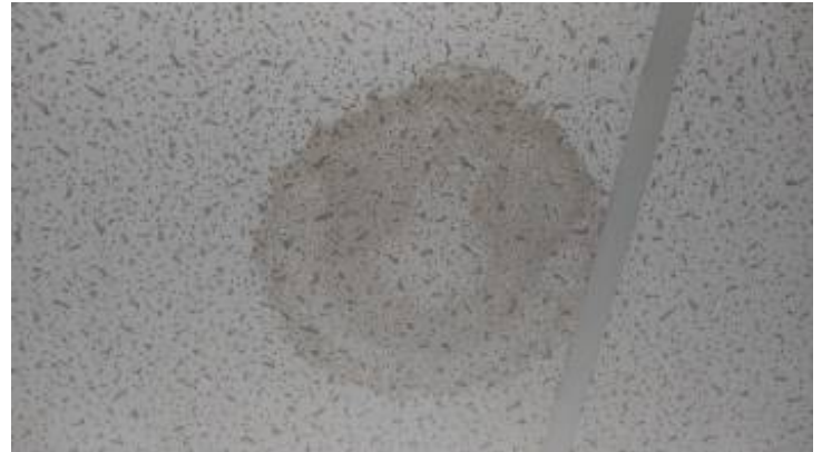
Very stained ceiling tiles I will note if they're still moisture.
