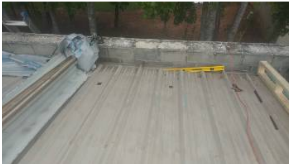
Needs a sloped roof going over the wall
