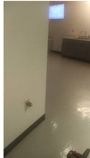
Outlet loose left side of the building
