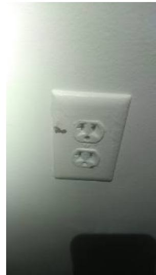
Painted receptacle in sanctuary not usable
