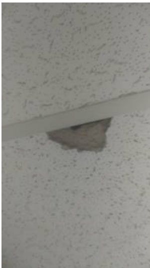
Several defects on ceiling tiles
