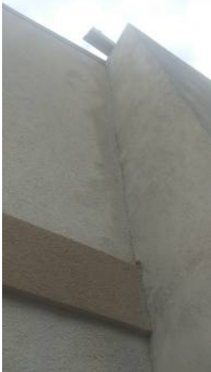
Signs of possible high moisture content
