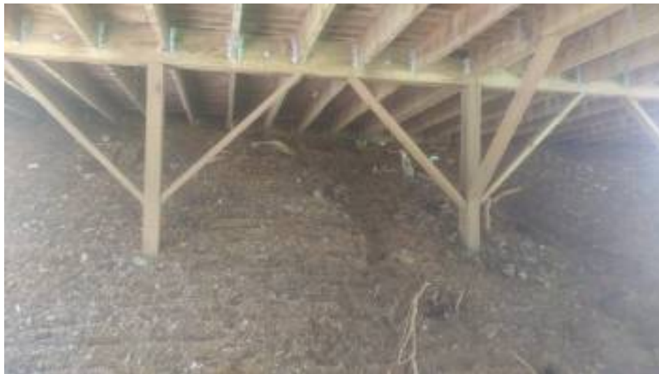
The large wood deck has a lot of wood to ground contact
