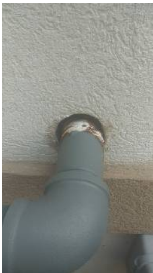
The opening around the gas meter piping should be sealed up.
