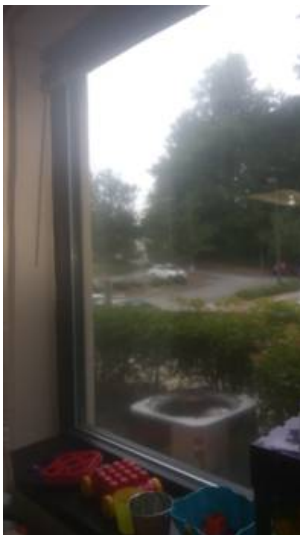
Broken seal in second child care room
