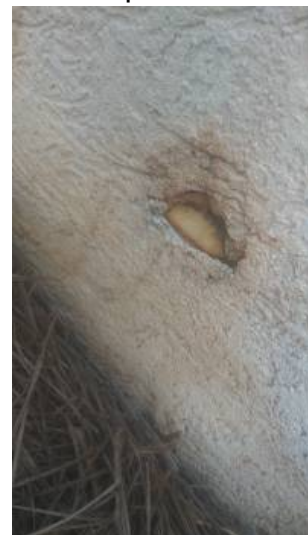
This is a sign that it does run underground have a qualified contractor repair
