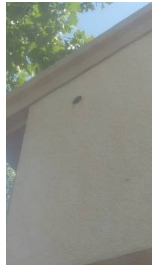
Whole should be repaired in back left corner
